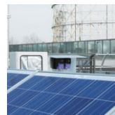
ITALY Cooling loop flow & temperature control
